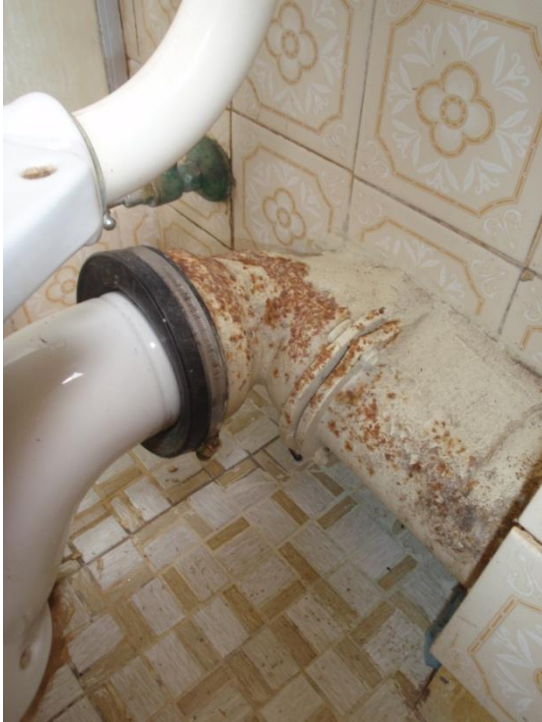
The Old and Unsightly Plumbing behind the Toilet
